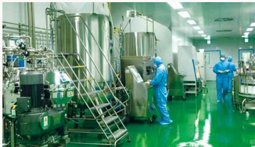
Cell-Culture Tanks at SK chemicals the Andong L House
